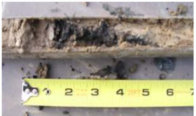
Figure 5: Vertical EHC fracture at 17 ft bgs (SB9).
