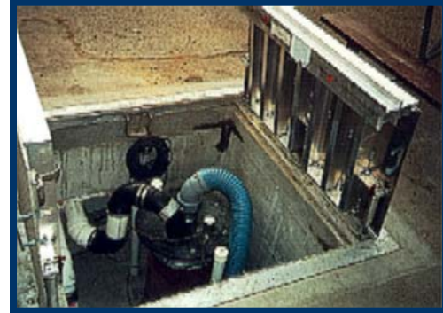
Vaulted system for BTEX/MTBE
