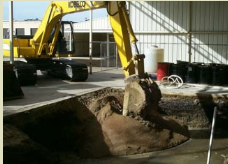
Figure 2. Placement of EHC and sand mixture at bottom of excavation to treat impacted groundwater following excavation of source area soil.
